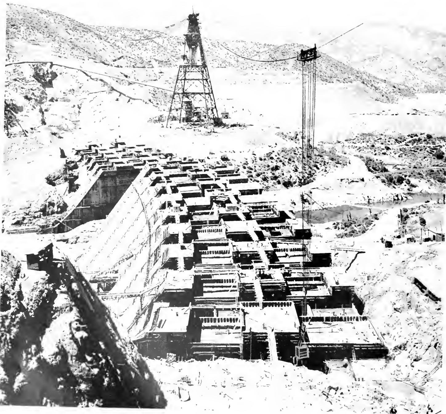
This view of Shasta Dam shows the progress of concrete pouring made to date by the cable system
